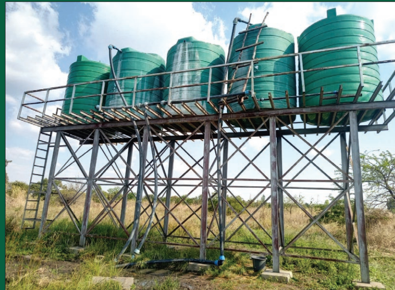
Two tanks added to existing three tanks to boost irrigation.
