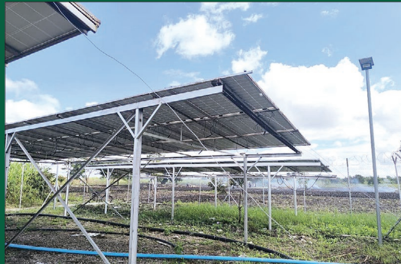
A solar panel field at Chome Irrigation Scheme in Phalombe District
